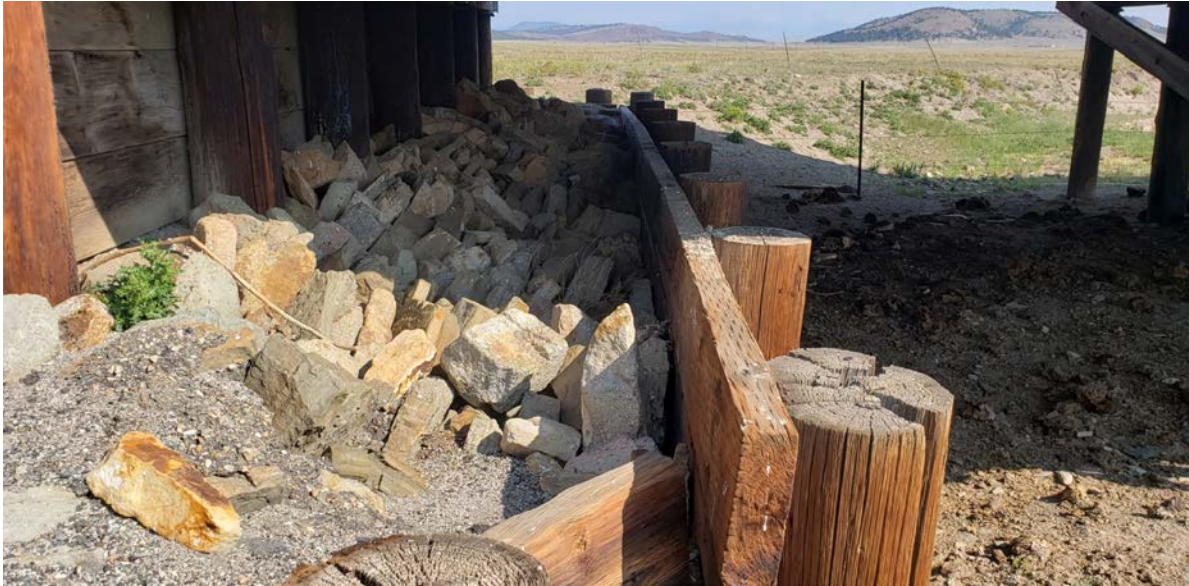
Picture 2 – Typical pile split and existing riprap
